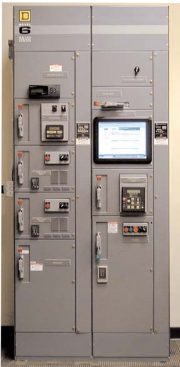
OMNI 6 MCC Cabinet
